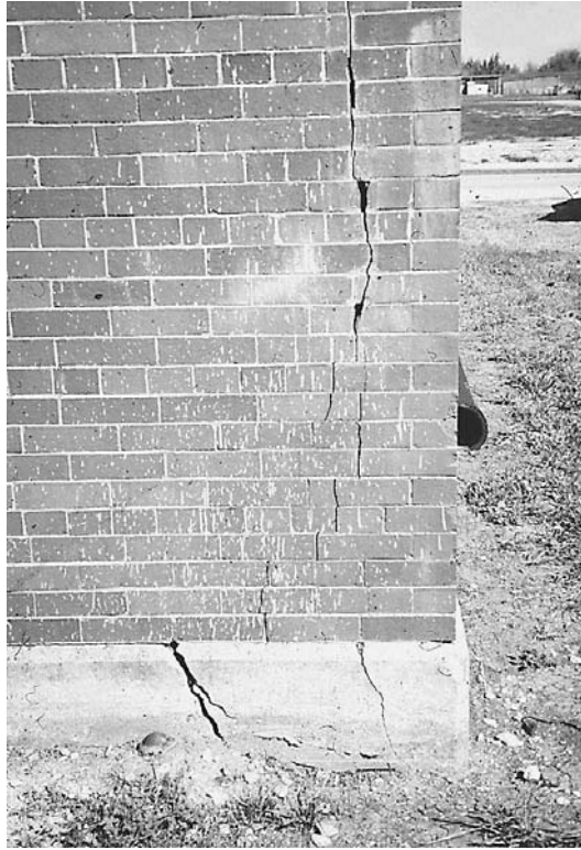
Figure 9-6 Opposing moisture expansion of brick and curing shrinkage of concrete slab can cause cracking at building corners if differential movement is not accommodated.
